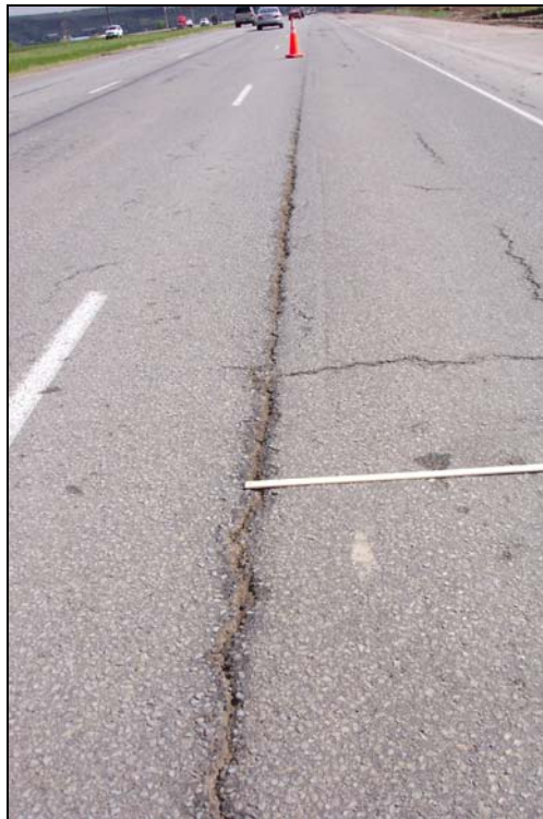
FIGURE 7: High Severity Longitudinal Cracking
