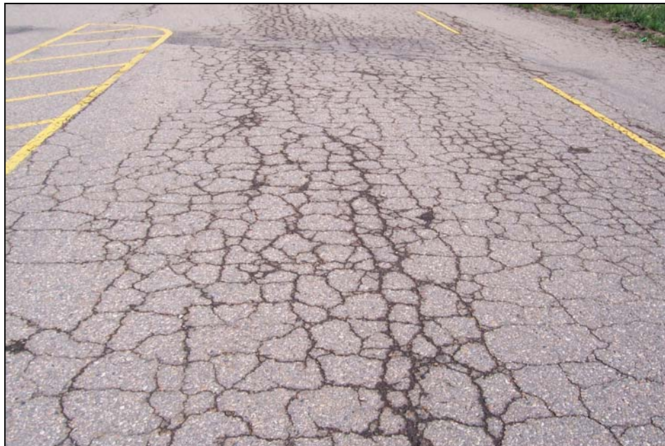
FIGURE 4: High Severity Alligator Cracking
