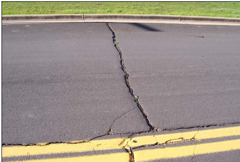
FIGURE 10: High Severity Transverse Cracking
