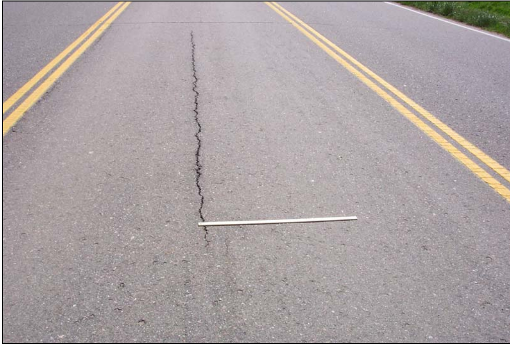
FIGURE 8: Medium Severity Longitudinal Cracking
