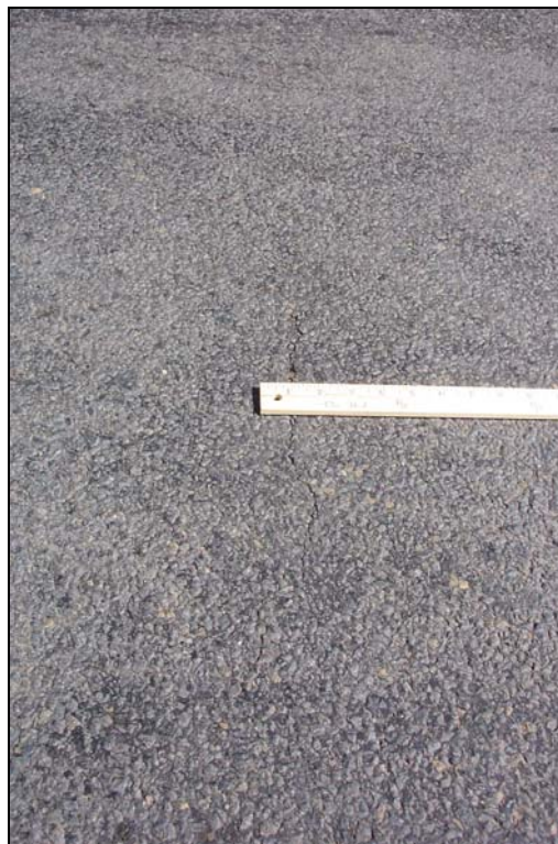
FIGURE 12: Low Severity Transverse Cracking
