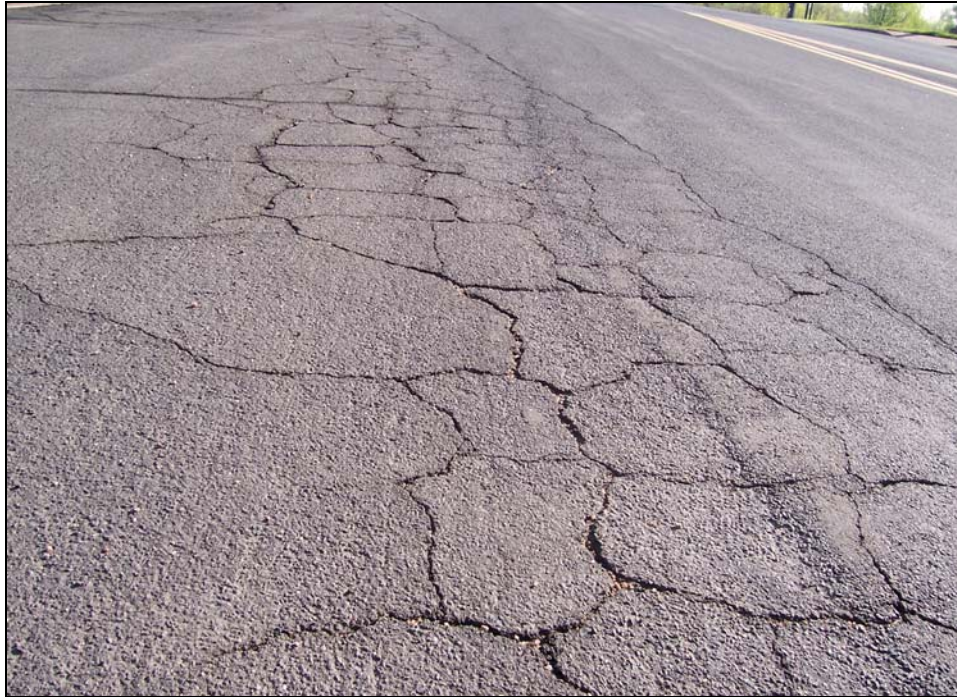
FIGURE 5: Medium Severity Alligator Cracking
