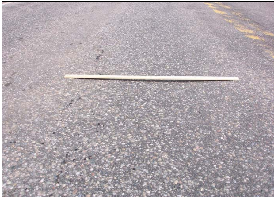
FIGURE 20: Medium Severity Rutting
