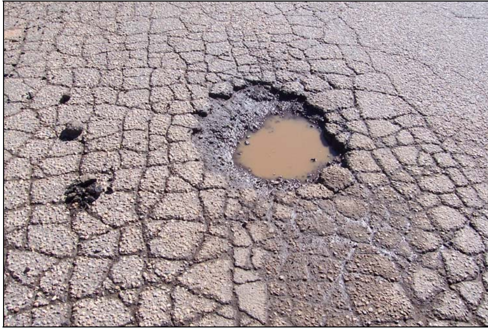
FIGURE 16: Pothole Surrounded by Alligator Cracking
