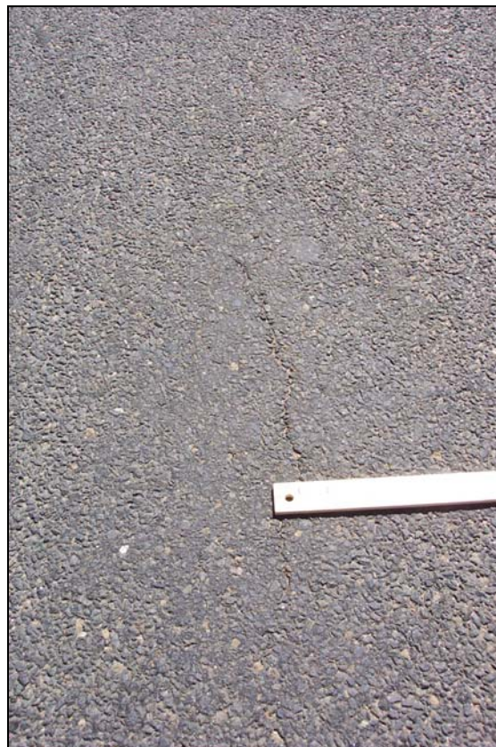
FIGURE 9: Low Severity Longitudinal Cracking
