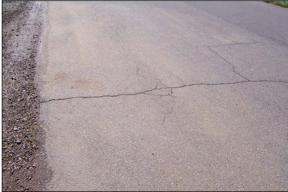
FIGURE 11: Medium Severity Transverse Cracking
