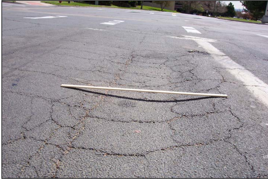
FIGURE 19: High Severity Rutting
