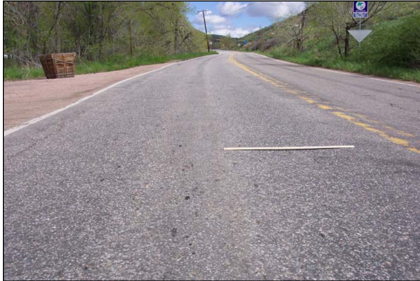
FIGURE 21: Low Severity Rutting
